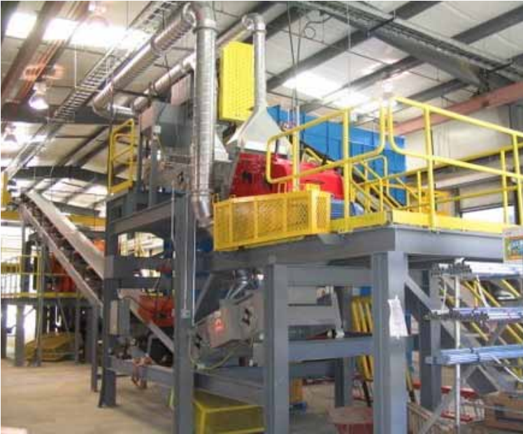
ERIEZ EQUIPMENT AT CRC FACILITY
