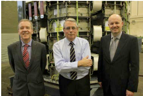
FaultCurrent's full-scale prototype during final assembly at Eriez' facility in Caerphilly, South Wales. In the foreground (left to right): FaultCurrent's Andy Cheer (COO), Martin Ansell (Chairman & CEO), Dr. Jeremy Hall (CTO)
