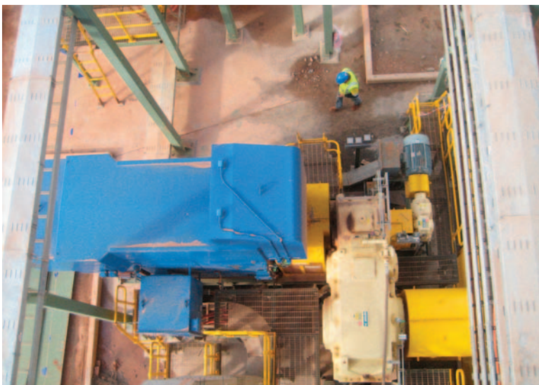
Overland conveyor drive motors.
