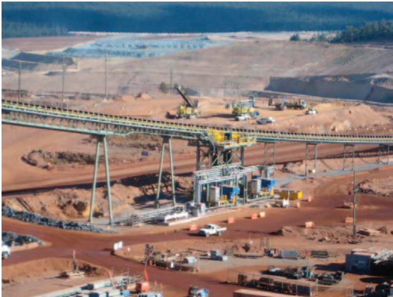
Overland conveyor drive system.
